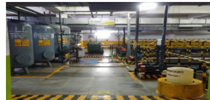
STP Plant 2*350 KLD
