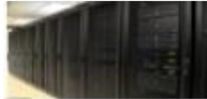
Modular UPS Efficiency 94%
